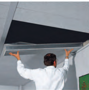
Typical suspended ceiling with removable insulated ceiling tiles
