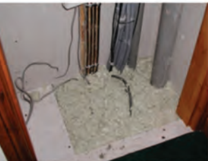
Incorrect use of 'foam' as a penetration seal. Courtesy of Siderise Ltd.
