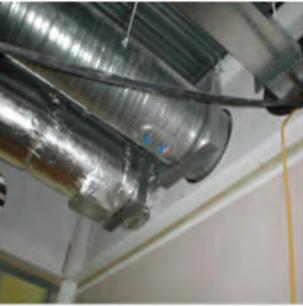
In this installation, the dampers are not in the plane of the wall, the duct is not protected and it is unlikely that the dampers have been tested in a cellular beam. Courtesy of Paul White.
