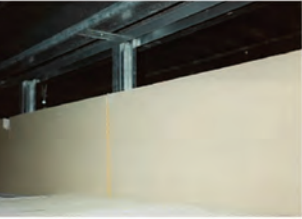
Vertical compartmentation not extending up to floor slab above (incorrect). Courtesy of Exova Warringtonfire.
