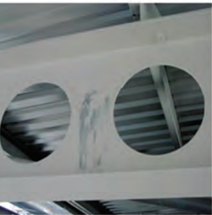
Slumping of intumescent paint on a cellular beam. Courtesy of Exova Warringtonfire Ltd.
