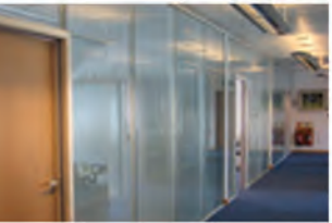
A typical fire resisting corridor with fire resisting glazing and doors.
