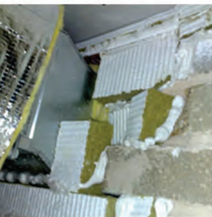
Poorly installed penetration seal to a damper. Courtesy of Exova Warringtonfire Ltd.
