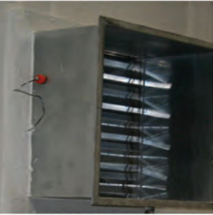
Fire damper correctly installed in the plane of the wall with no damage to the penetration seal. Courtesy of Paul White.
