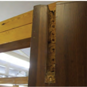
voids in a fire door. Courtesy of Chiltern Fire/BM TRADA.
