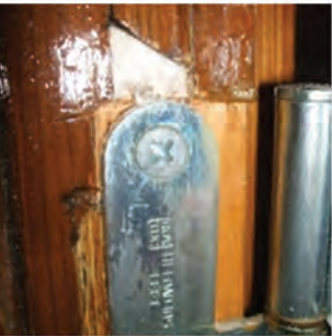
Replacement hinge badly fitted to door. Courtesy of Guild of Architectural Ironmongers.
